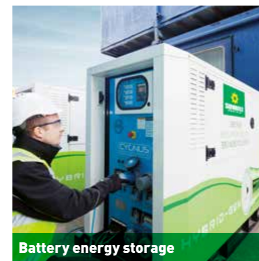
Stage 5 low emission generators
